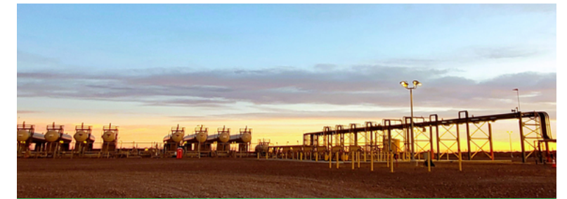
Diamond NGL Facility
